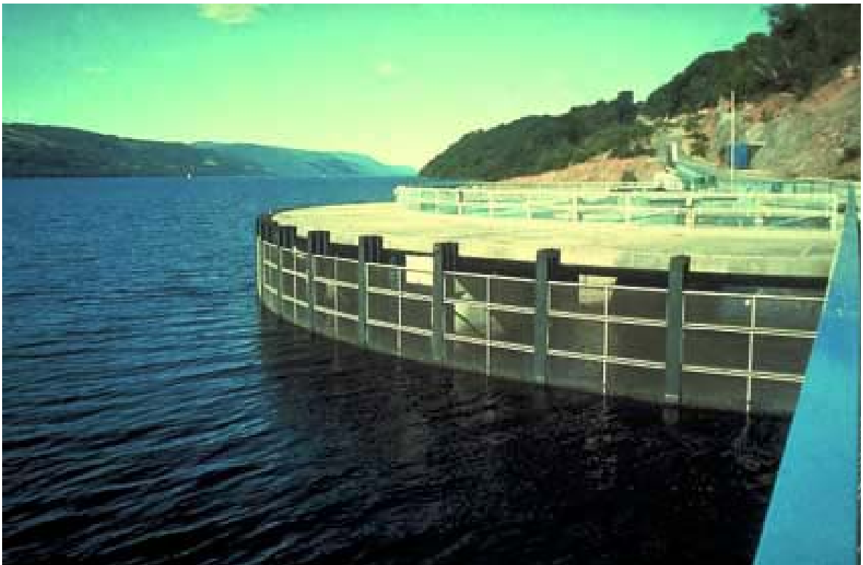
Photo 24: Fine mesh screen at an hydroelectric power plant intake on the Loch Ness in Scotland. (Photo Travade)
