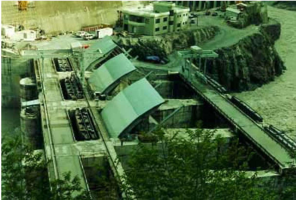
Photo 3: The 44 m high Kali Gandaki “A” Hydroelectric Dam (Nepal), which was still under construction in 2001, cuts off local fish species, e.g. Tor sp. and Bagarius bagarius , from their valuable spawning grounds upstream. (Photo Marmulla)
