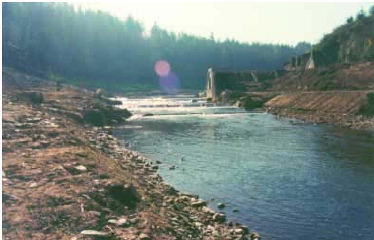
Photo 29: The 15 m high Kernansquillec dam was decommissioned and destroyed in 1996 to restore the ecological quality, particularly the salmon population, on the Leguer river (Britanny, France). (Photo Larinier)
