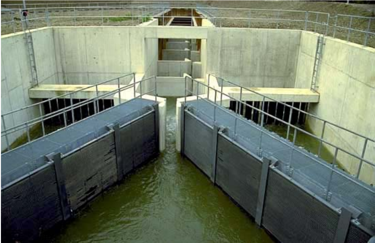
Photo 21: Introduction of auxiliary water through lateral screens at Iffezheim fish pass (river Rhine). Auxiliary flow is supplied from forebay through a special turbine (fish pass discharge 1.2 m 3 /s, turbine discharge 12 m 3 /s). (Photo Larinier)
